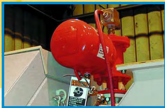
Air Cannons are mounted at the intake and discharge to help prevent build up of wet material.
